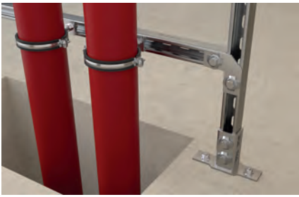
Waste water pipe
