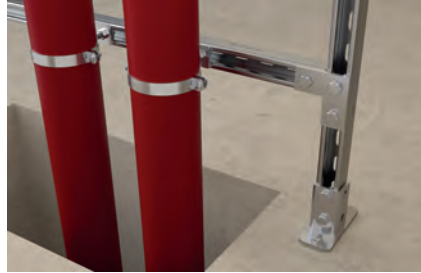
Waste water pipe
