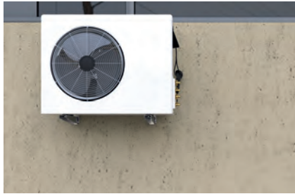
Airconditioner on the outer wall
