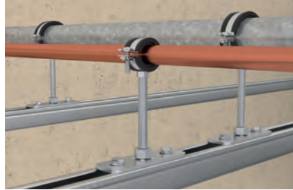
Baseplate on installation channel
