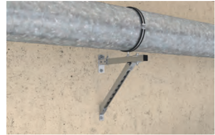
Spiral airduct on cantilever
