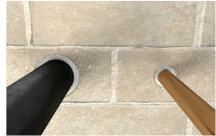
Non combustible services
