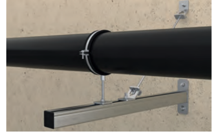
Heavy pipe on cantilever
