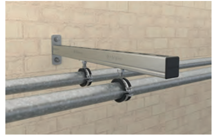
Pipelines on cantilevers
