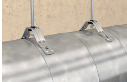
Spiral duct pipe with sound insulated hanger
