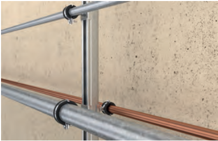
Lateral pipe mounting at channel
