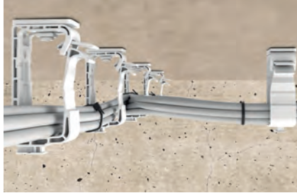
Bundling electric cables
