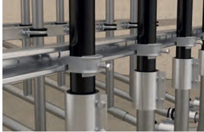
Supply lines fixed to FUS channel
