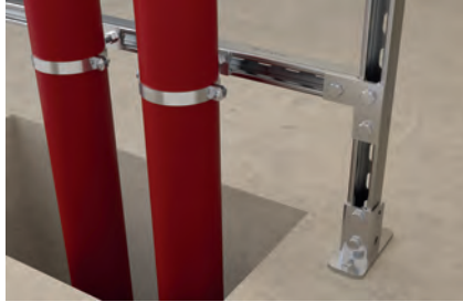
Waste water pipe
