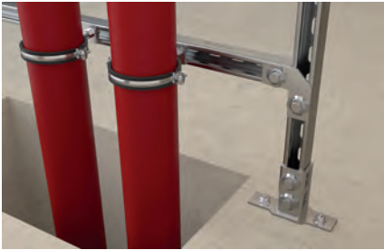
Waste water pipe
