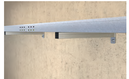
Cable tray on cantilever arm
