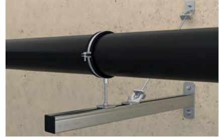
Heavy pipe on cantilever
