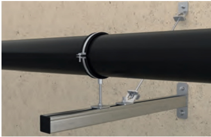
Heavy pipe on cantilever
